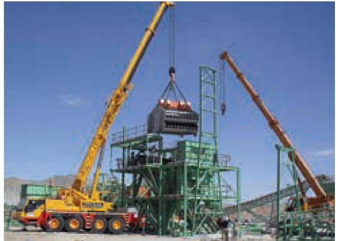
Joest vibrating screen being installed at the Navachab gold mine in Namibia.
