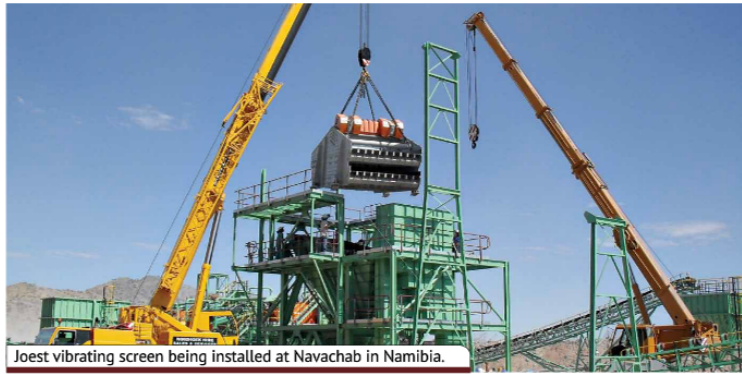
Joest vibrating screen being installed at Navachab in Namibia.
