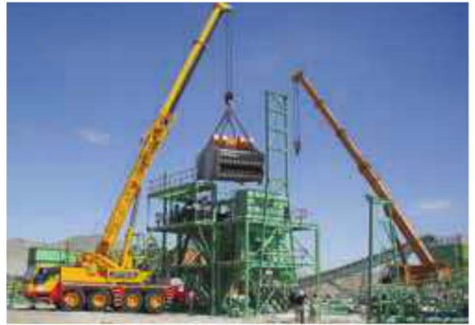
A Joest vibrating screen being installed at a gold plant in Namibia.
