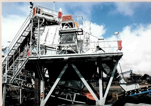
A Joest Kwatani coal plant primary feed sizing screen.
