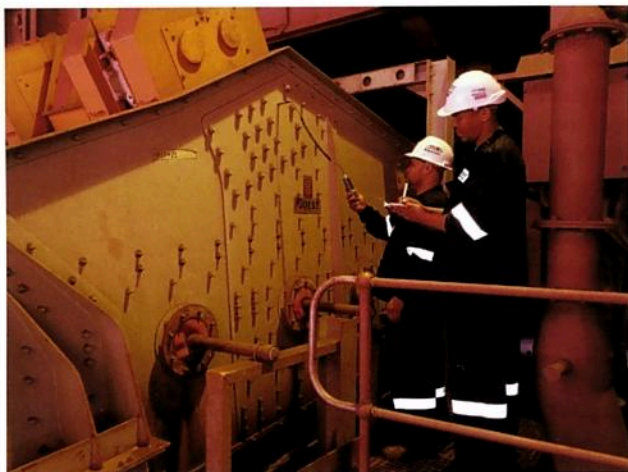
Equipment auditing including periodic condition monitoring is used to assess the status of a screen at a point in time
